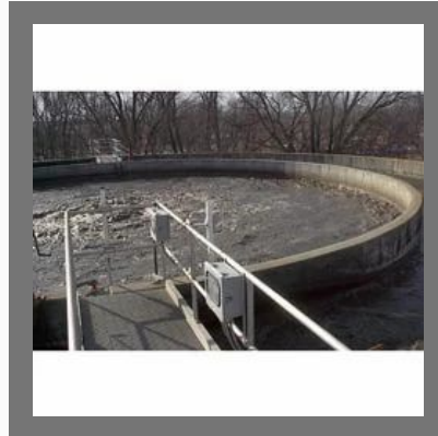
Sewage Treatment Plants
