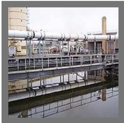
Effluent Treatment Plants
