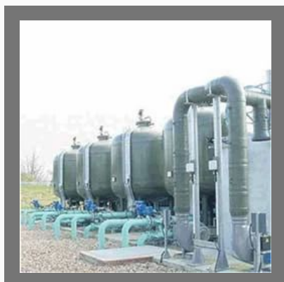
Water Treatment Plant Consultancy Services
