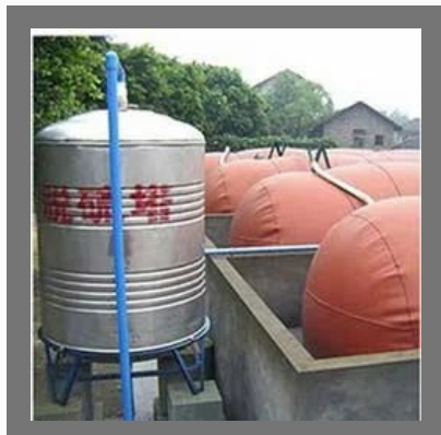
Industrial Biogas Plants
