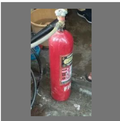
Fire Pro Extinauishers
