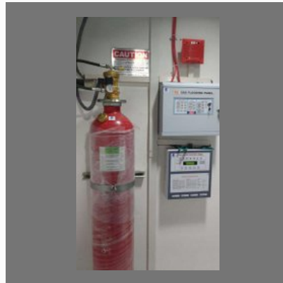
FM 200 Fire Suppression System
