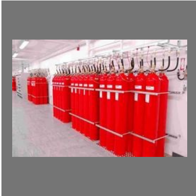
Fire Suppression System
