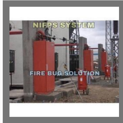
Nitrogen Injection Fire Protection System
