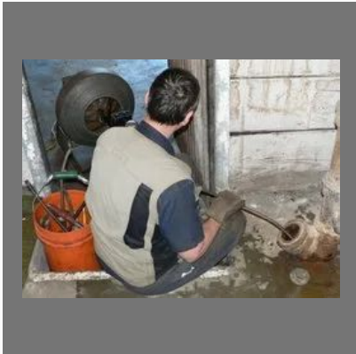
Drain Sanitary Plumbing Services
