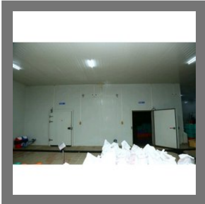
Cold Storage Room
