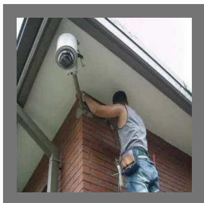
Maintenance CCTV Camera Service
