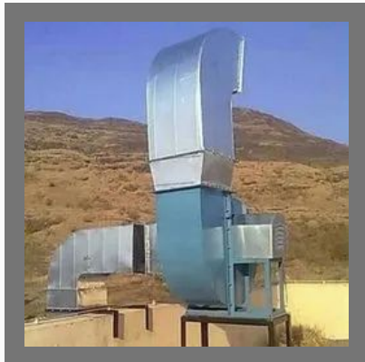
Stainless Steel Duct
