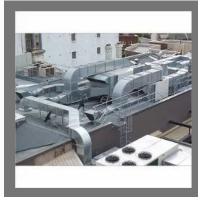
Industrial Air Duct
