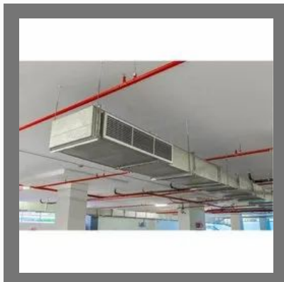
Ceiling Duct AC
