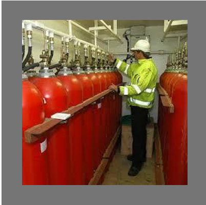
Inspection Of Fire Fighting Installations
