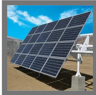
Surface Solar Power Plant
