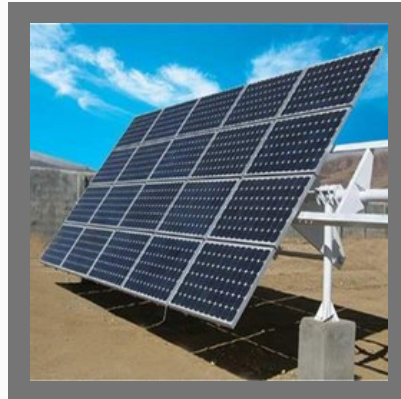
5KVA Solar Power System
