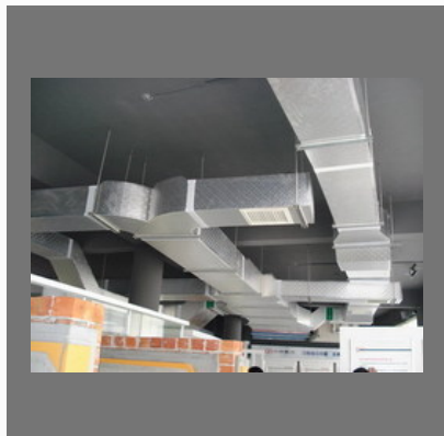
Preinsulated AC Ducting
