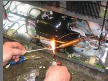
Refrigeration Repair And Service
