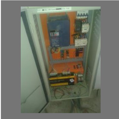
Elevator Control Panel
