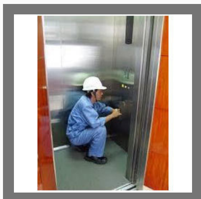
Elevator Maintenance Services
