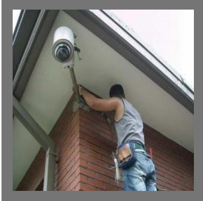
CCTV Camera Installation Services
