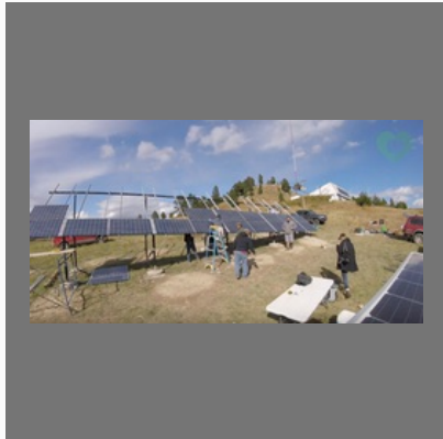
Solar Epc & Bos Services
