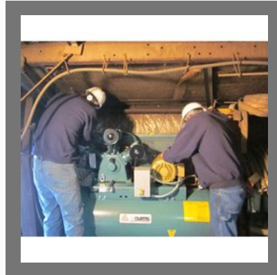
Air Compressor Maintenance Service
