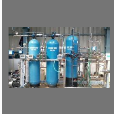
DM Water Plant
