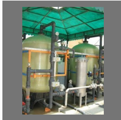
High M3 DM Plant For Boiler Feed Water
