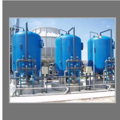
Iron Removal Plant
