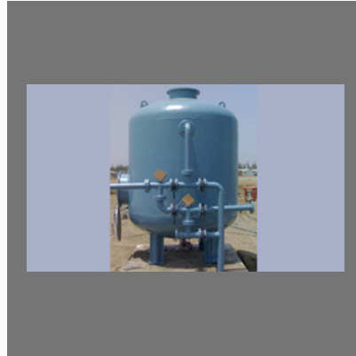
Arsenic Removal Plant
