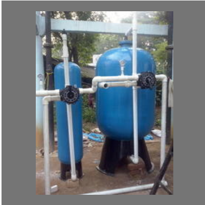
Iron Removal Plant
