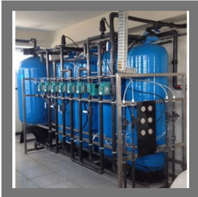
HCL Added Water Treatment Plant
