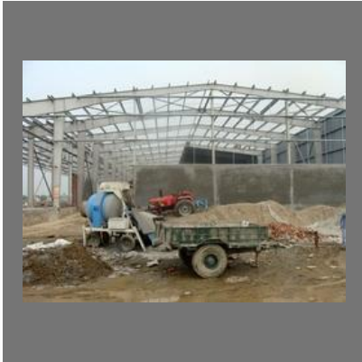
Pre Engineering Building Services
