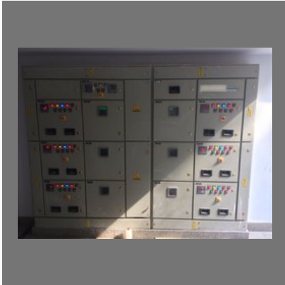
LT Panel/MCC/APFC/Distribution Panel
