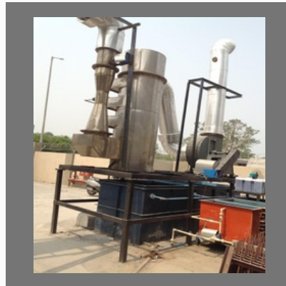
Retrofitted Emission Control Equipment
