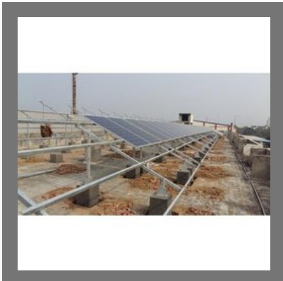
Off Grid Solar Power Plant
