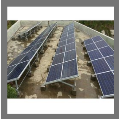
Rooftop Solar Power Plant
