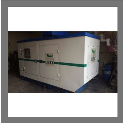
380 kVA Kirloskar Silent Generator
