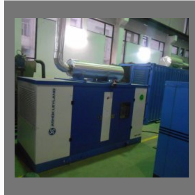
62.5 KVA Ashok Leyland Gas Genset
