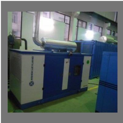
Gas / Png Generators
