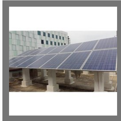
On Grid Solar Power Plant
