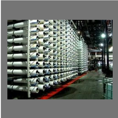
Reverse Osmosis Systems
