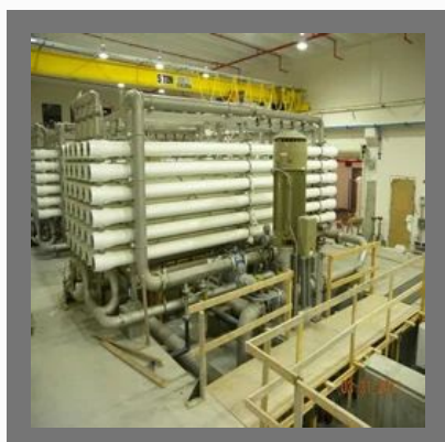
Sea Water Desalination Plant
