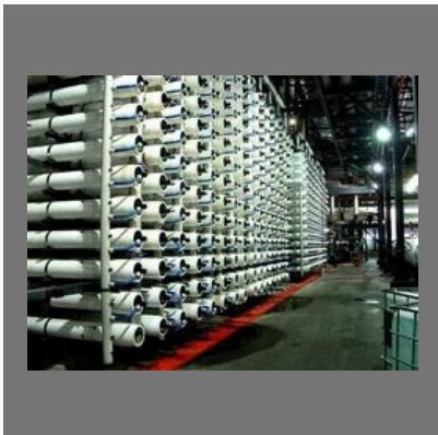
Industrial Reverse Osmosis Plant
