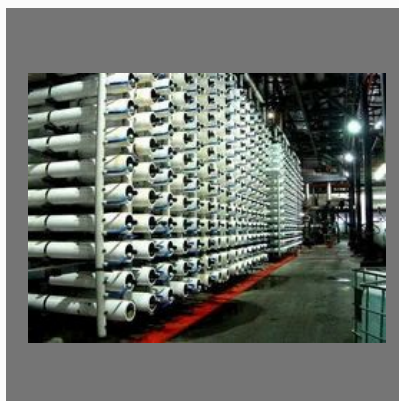
Reverse Osmosis Equipments
