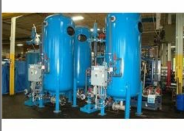
Water Softener Plant
