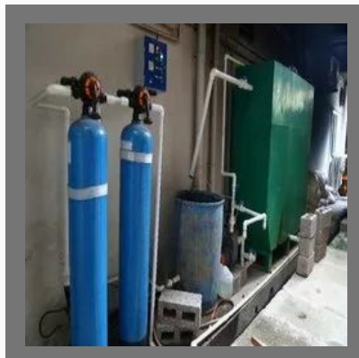
Domestic Sewage Treatment Plant
