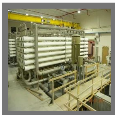
Sea Water Plant
