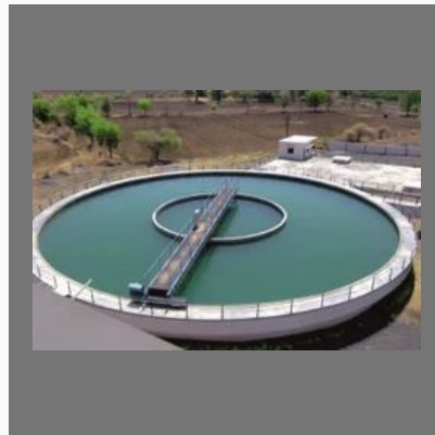
Automobile Effluent Treatment Plant
