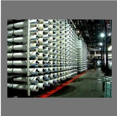
Reverse Osmosis Plants (RO)
