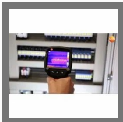
Thermography Electrical Panel
