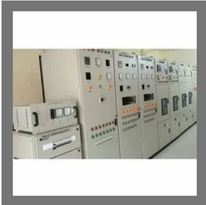
Main LT Three Phase Control Panel
