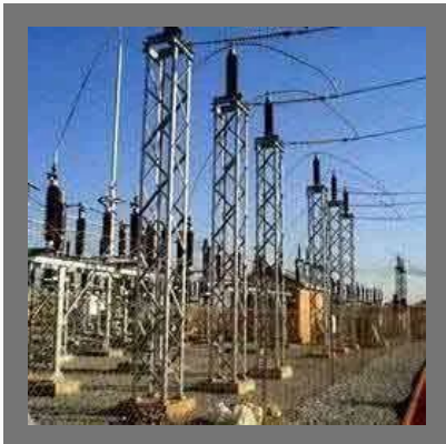
HT / LT Installations Services
