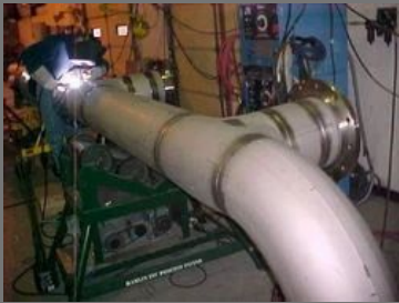
Pipe Fabrication Service
