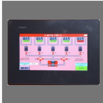
Automatic Condenser Tube Cleaning Control Panel
