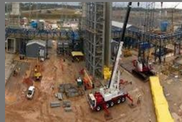
Power Project Services
