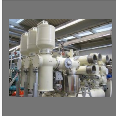
Gas Insulated Switchgear
