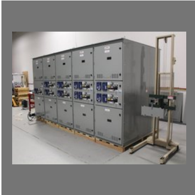
Medium Voltage Switchgear - VCB - Eaton Make
