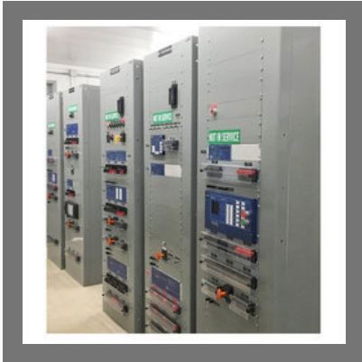
Relay Control Panel
