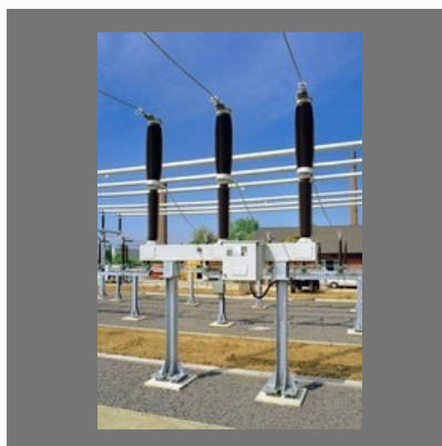
SF6 Circuit Breaker
