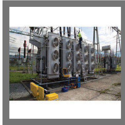
Relay Testing - Training
