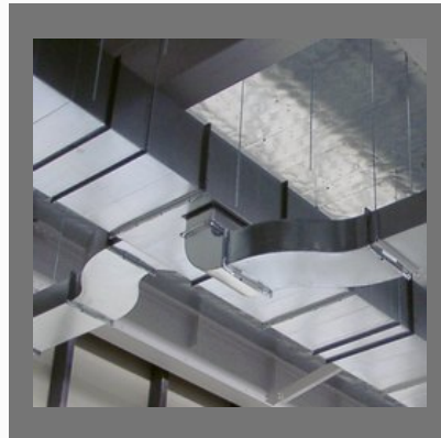
Carrier HVAC Duct
