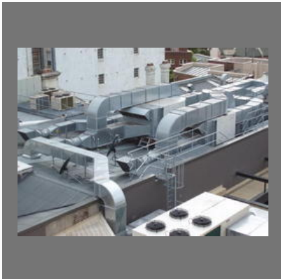
Hitachi HVAC Duct
