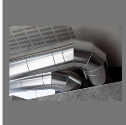
Blue Star HVAC Duct
