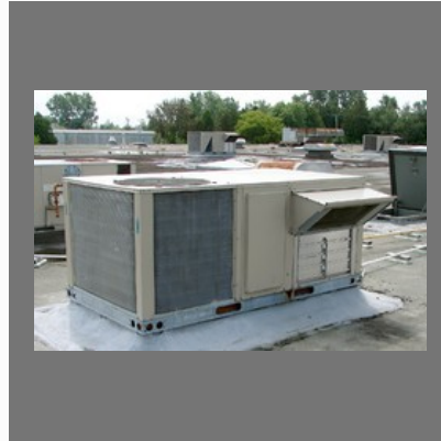
Blue Star HVAC System
