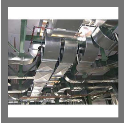
Daikin HVAC Duct
