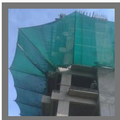
Building Safety Nets
