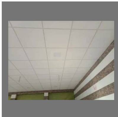
Mineral Fiber False Ceiling
