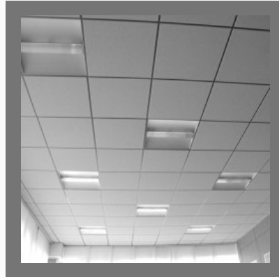
PVC Grid False ceiling
