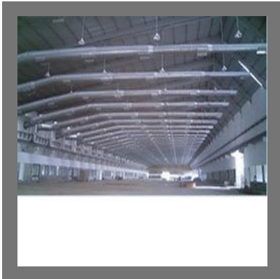
Insulated Spiral Duct
