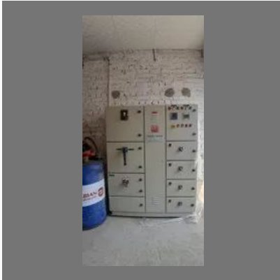
Electrical Control Panel
