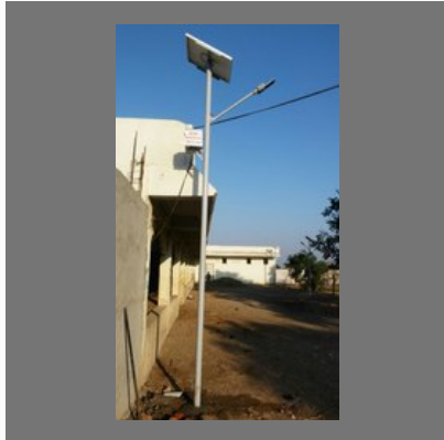
Solar Street Light
