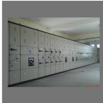
Medium Voltage Panel
