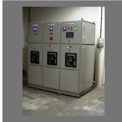
AMF Control Panel
