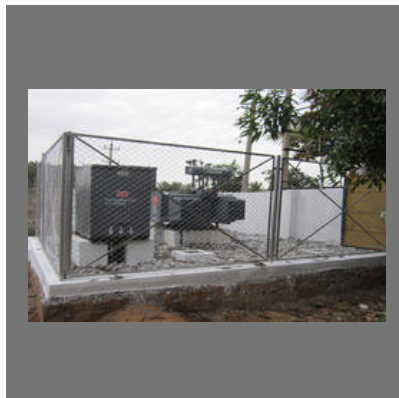
Electrical Power Panel
