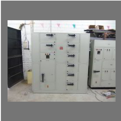
Sub Switch Board
