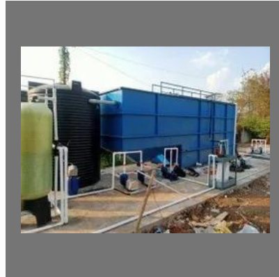
Sewage Treatment Plant
