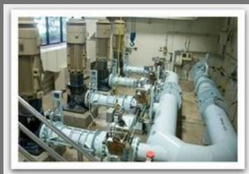
Industrial Sewage Treatment Plant
