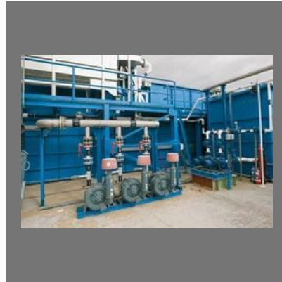
STP Engineering service
