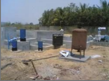
ETP Commissioning Service
