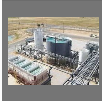
Zero Liquid Discharge Plant
