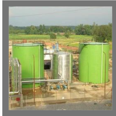
DM Plant Engineering service
