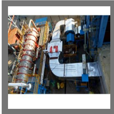
Gas Heat Exchanger
