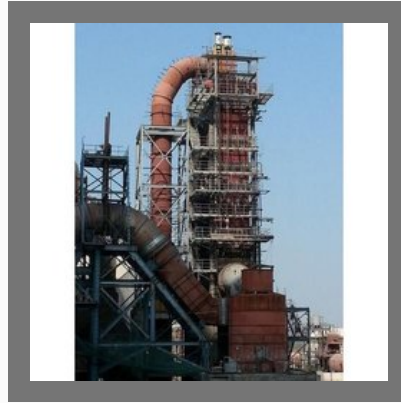
AQC and PH Boiler
