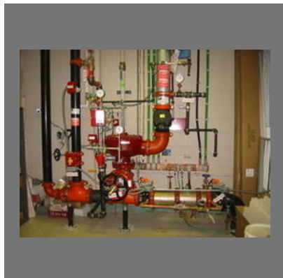
Fire Detection And Protection Project
