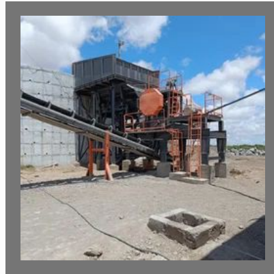
Stone Crusher 150 Tph
