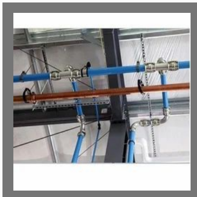
Compressed Air Aluminum Piping
