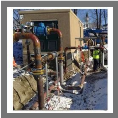
Fuel Utility Piping Turnkey Projects
