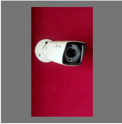
Window CCTV Camera
