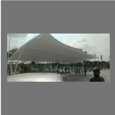
Fiber Car Parking Sheds
