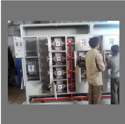
Electrical Distribution Panels
