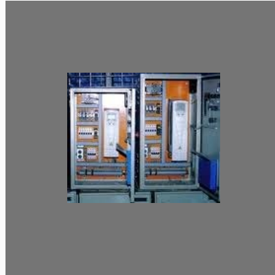
VFD Control Panels
