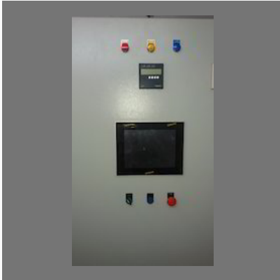
Automation Control Panels
