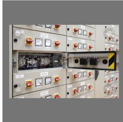
Electrical Power Panels
