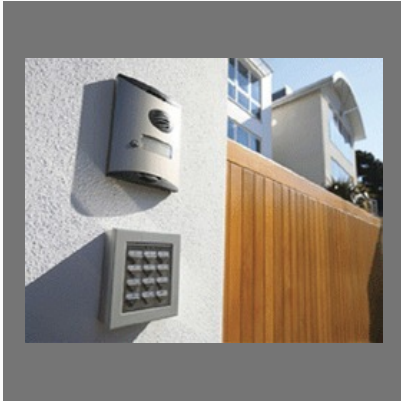
Access Control System
