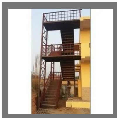
Mild Steel Staircase
