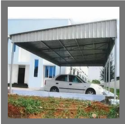
Mild Steel Car Parking Shed
