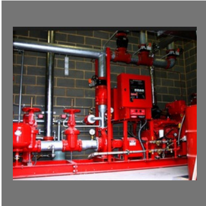
Fire Hydrant System
