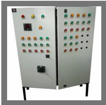
Mild Steel MCC Power Panel
