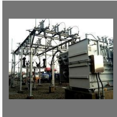
Substation Electrical Contractor
