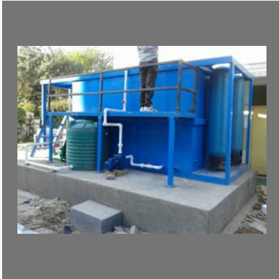
Sewage Treatment Plants
