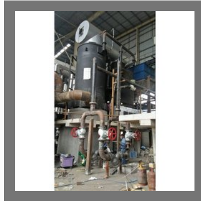
Thermic Fluid Heater
